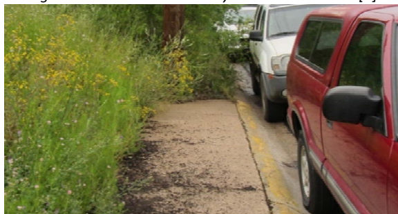
Figure 9 Eastside sidewalk conditions [4]
